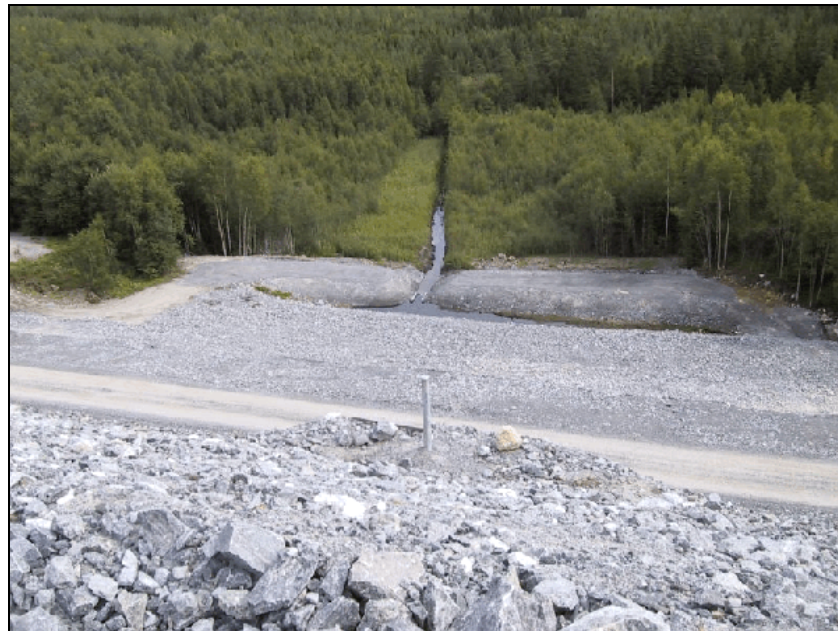
Figure 3.23: Another ditch for collection and flow measuring of seepage water alongside the dam [66, Base metals group, 2002]
